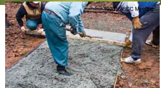
Once enough concrete is in the form, use 2x4 to screed, filling all areas.
