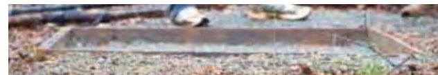
A level form is best for sure footing. At or slightly above grade is ideal.
