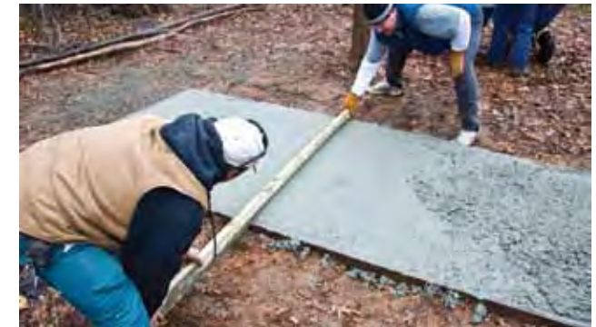
As you screed, you may need to fill in low areas with excess concrete.
