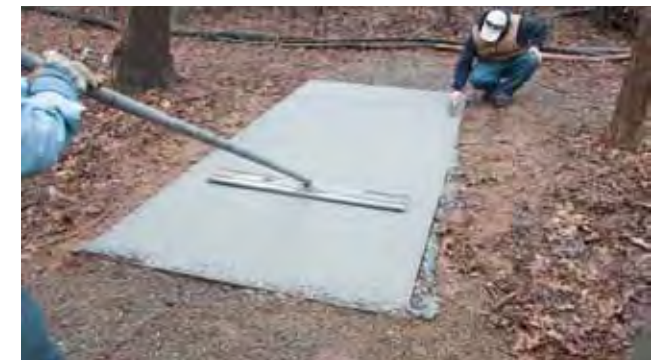
Float the concrete to force rocks down. It will help with texturing.
