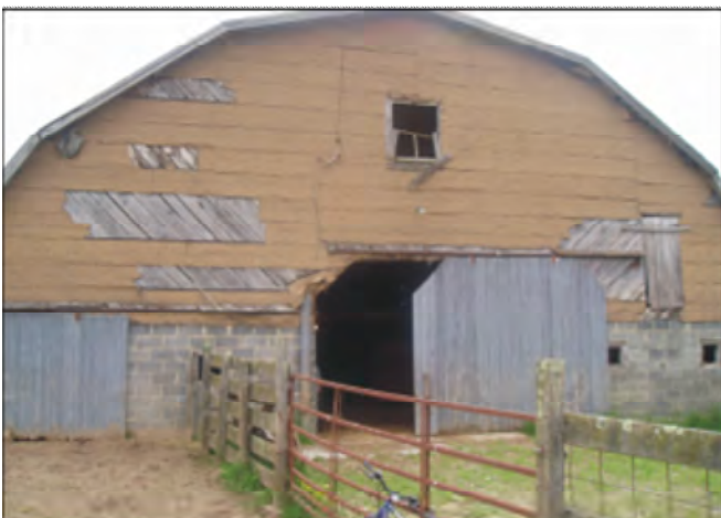
Photo Three: View of structure number 3, pole barn, built in the 1950's.
