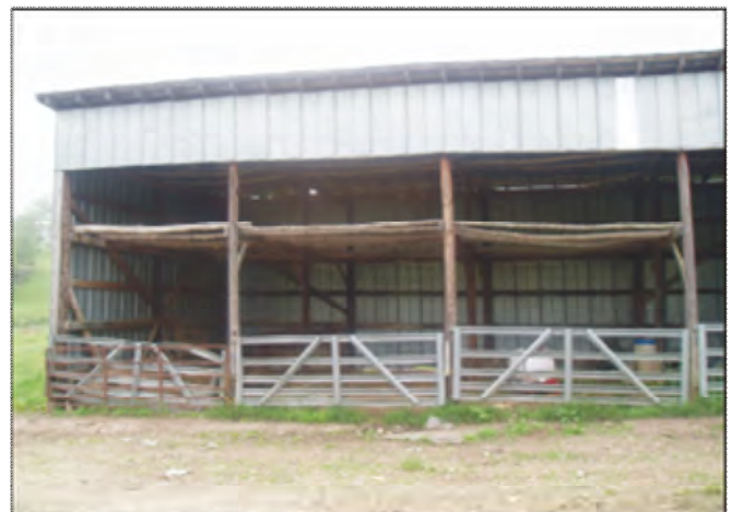
Photo Four: View of structure number 4, pole barn, built in the 1960's
