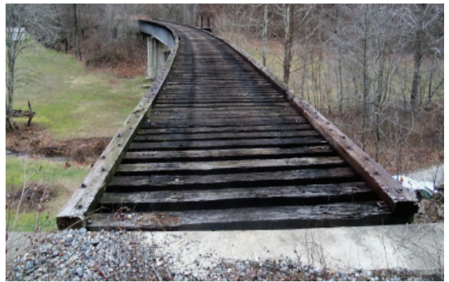
Dawkins Line - Rails to Trails Johnson, Magoffin & Breathitt Counties, Kentucky Before Construction
