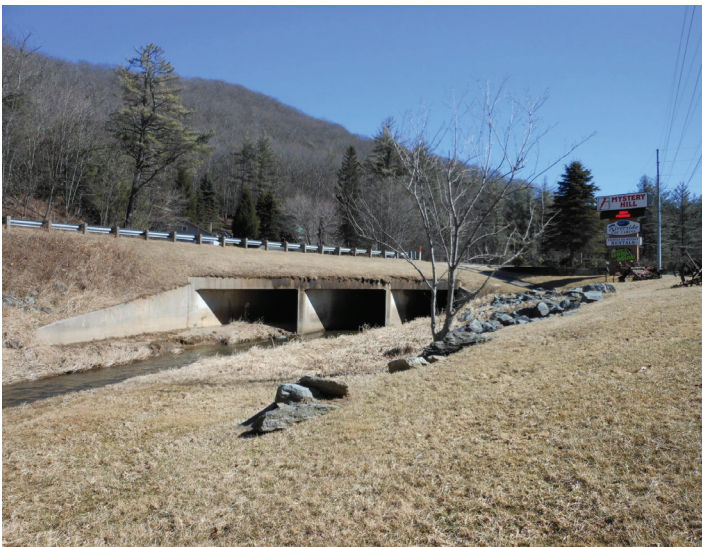
Existing Culvert Crossing - The proposed trail will go under existing US 321 inside this culvert.
